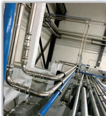
● Cooling water for Auto Parts.
