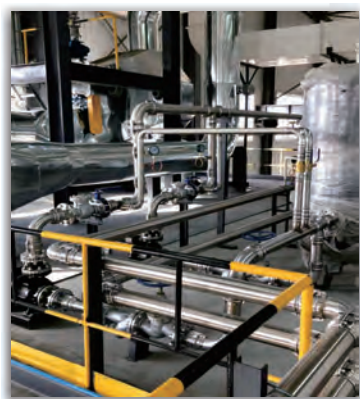
● Cooling water for new Material.
