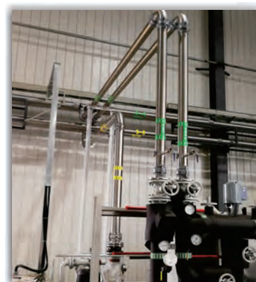
● Oil and Cooling water for Machinery.
